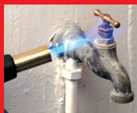
Thawing frozen pipes
